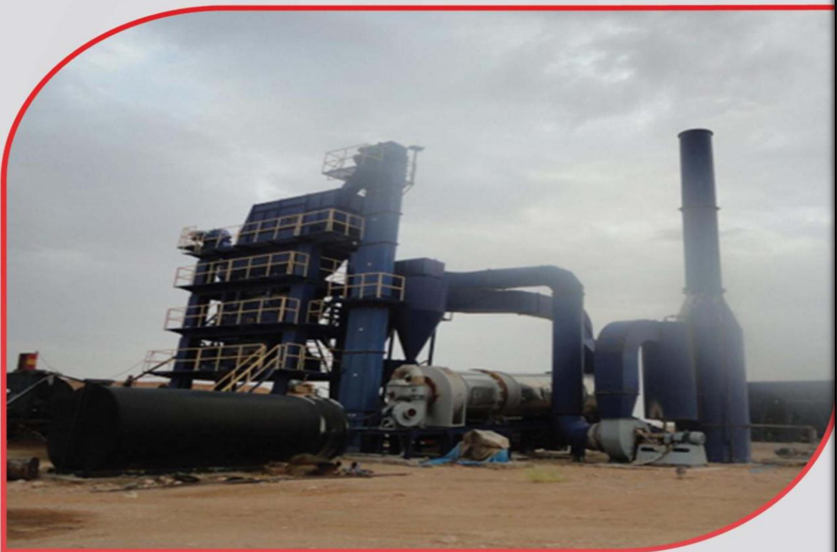
These Photos are for the YHC Asphalt Mixer at Ataq Base Camp in Shabwah Governorate.
